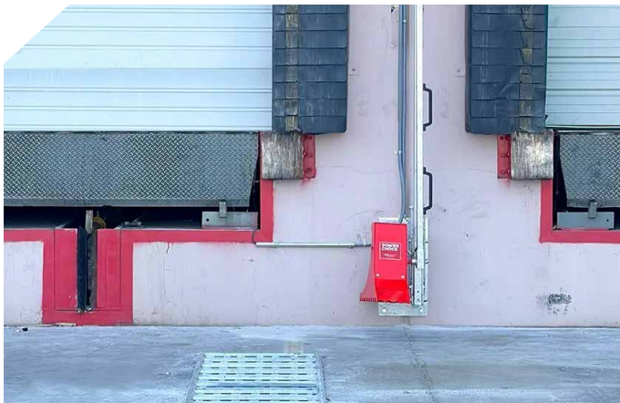
SGWS facility in Las Vegas – Installation in 2021.
