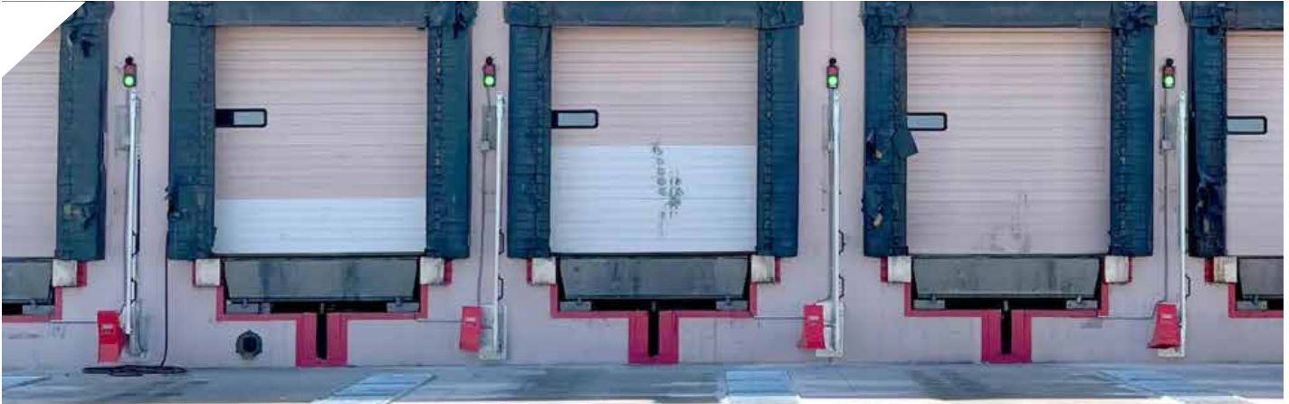
SGWS facility in Las Vegas - Installation in 2021.
