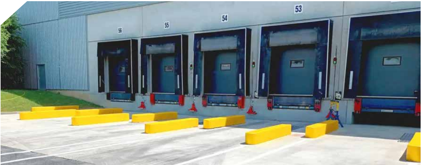
The 81 loading docks of the logistics facility in Brie-Comte-Robert are secured with the portable vehicle restraint POWERCHOCK 3.
